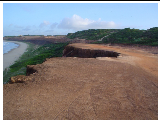
Figure 8. Gully at the crest of a sea cliff at South Sector.
