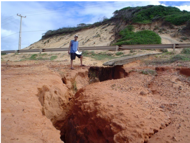
Figure 5. Erosion at the top of a sea cliff in North Sector, caused by rainwater discharge.
